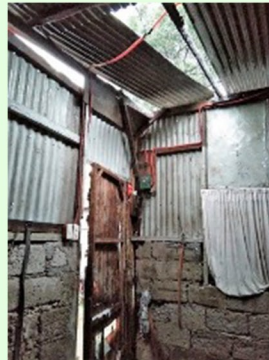
Damaged door & roof of the Mortalla house in SJDM, Bulacan
